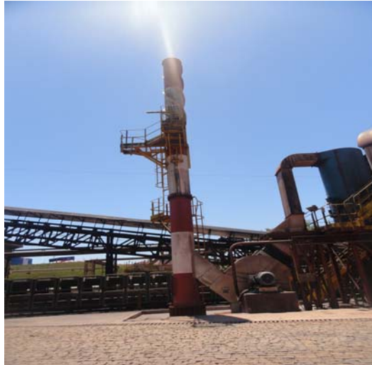
Figure 7 Dust collector (photo of the author's field visit)
