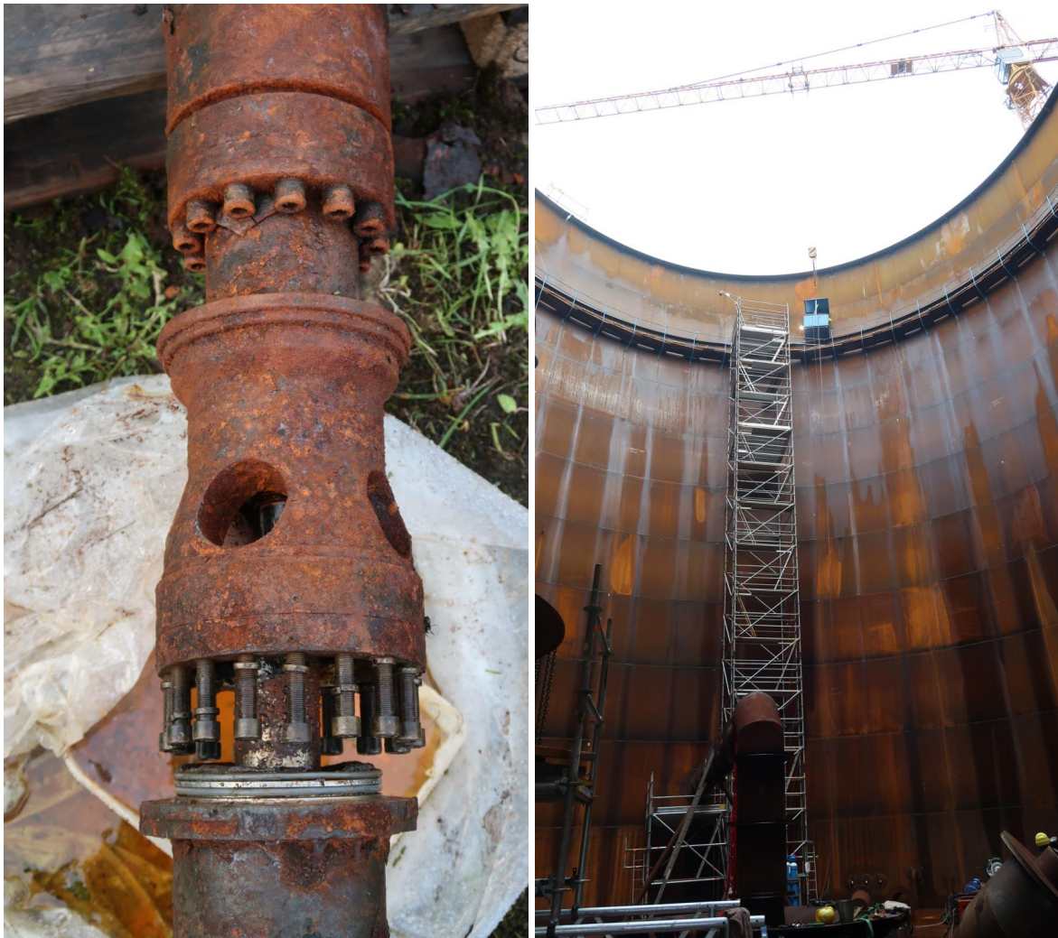
Figure 4.6: Left: Corroded well pump of the cold well of the HT-ATES in Neubrandenburg. Right: Artificial storage tank to balance short-term supply-demand mismatch.
