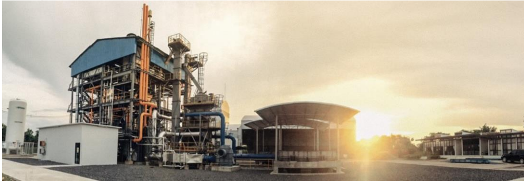
Figure 4. DFB gasification power plant at Nongbua district, Nakhon Sawan province, Thailand
