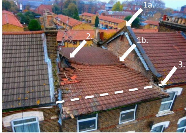
Figure 1: The collapse of a roof in Tottenham, U.K., 2014. Picture from http://www.tottenhamjournal.co.uk/news/lunchbreak_saves_lives_of_builders_in_tottenham_roof_collapse_1_3858222 .
