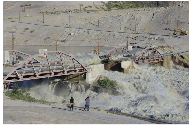
Figure 2. Photograph taken at 18:00 West Greenland Summer Time on 11 July 2012 during the flood with the Watson River Bridge being washed out. Image courtesy of Jens Christiansson.
