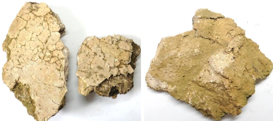
Plates No. 1 & 2: The left plate shows the intact pieces in the plaster sample, as-received, with the outer finish coat in view. It was noted that cracks in the finish coat are highlighted by entrapped soiling and algal growths. The right plate shows an internal, masonry contact surface of the inner base coat plaster, with adhered soiling. The soiling is clayey to touch and may infer that the masonry was either bedded in a clay or clay lime mortar, or the interface was exposed to weathering with decay of the plaster at the masonry interface.
