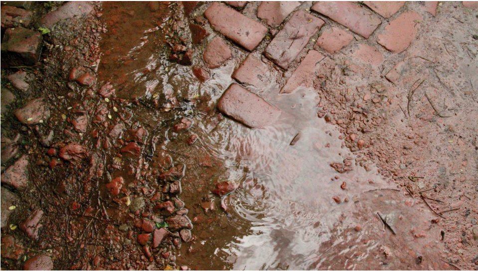
Figure 6. Weathered road surface and disintegrated bricks. Credit: Author.
