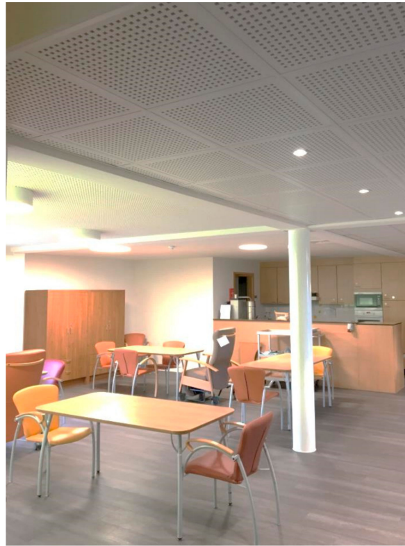
Figure 5. Picture of the nursing home (NH) living room after the installation of the acoustic floating floor and absorbing ceilings.
