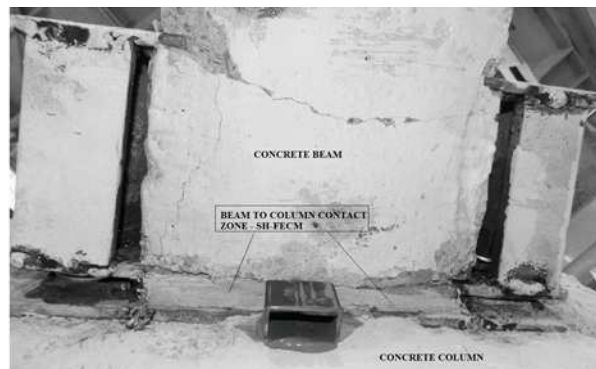
Figure 2 Hybrid spatial joint model after testing - critical interface zone, bottom view: good performance of SH-FECM, no spalling or large visible cracks
