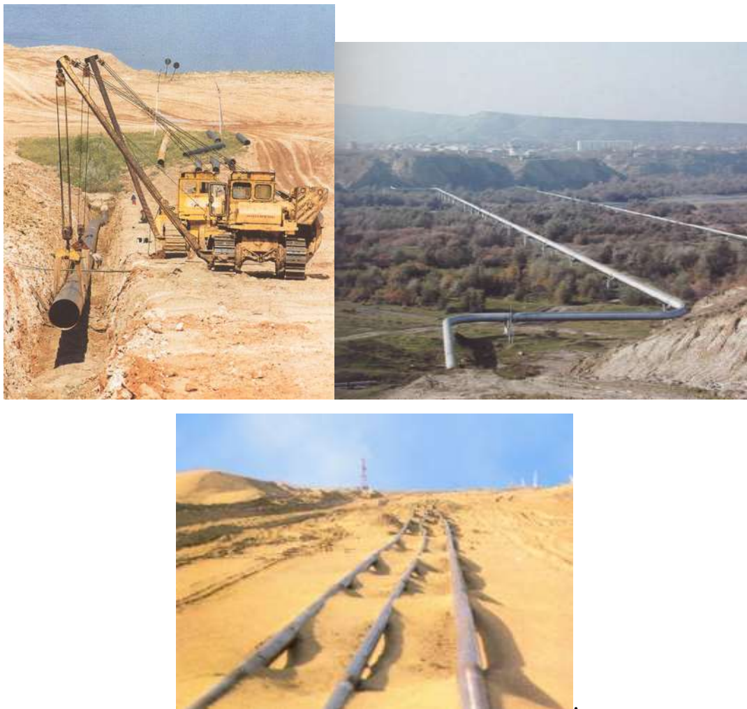
Figure 33 – Methods of pipelaying: underground (top left), above-ground (top right) and on-ground (bottom) [2]
