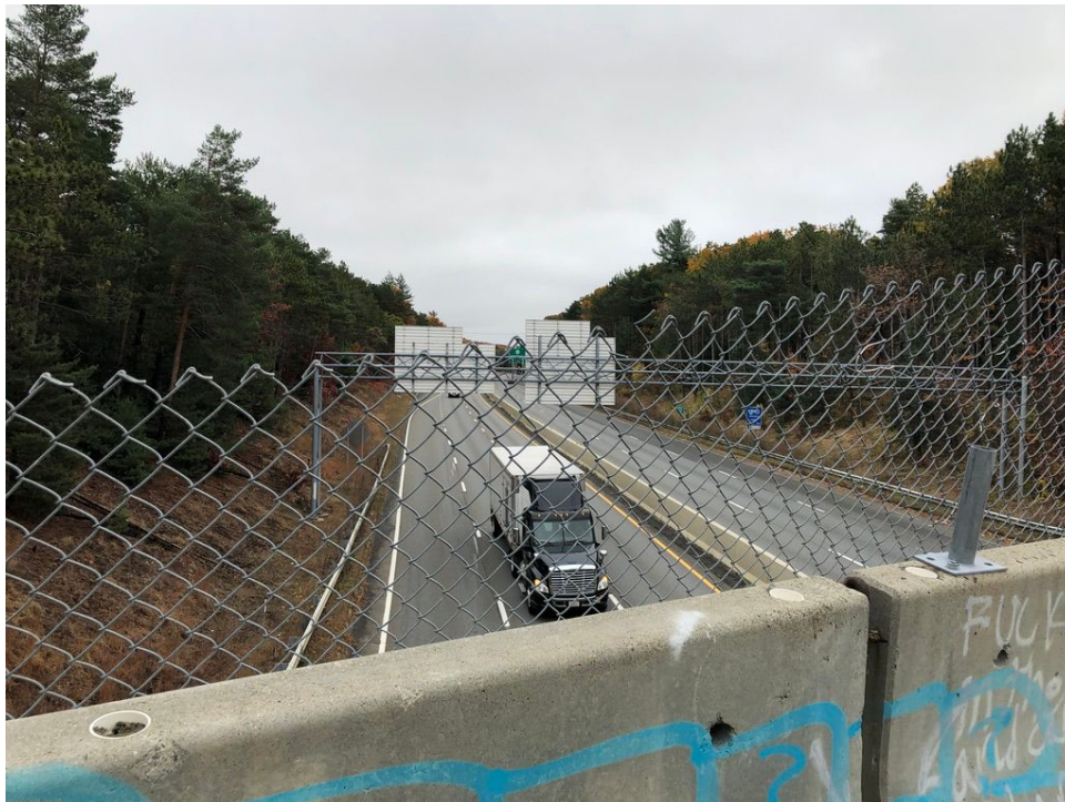
Photo 6: View from bridge looking east onto Route 2 over collapsed fence.
