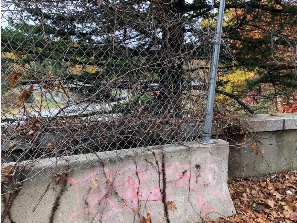
Photo 9: Tree overgrowth onto structure, looking west.
