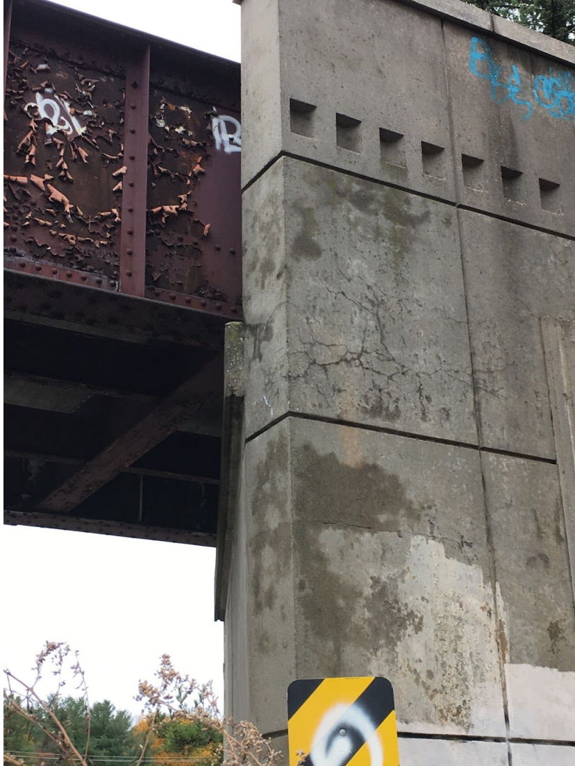
Photo 13: Looking west, map cracking on north bridge abutment.
