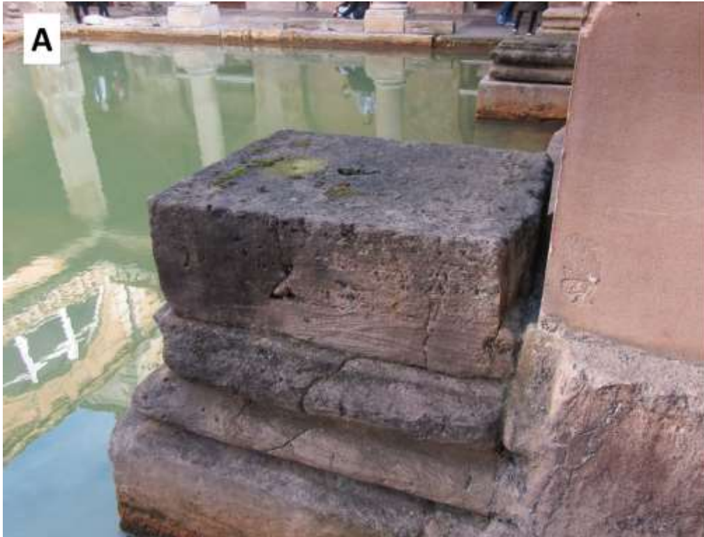
Figure 4. A: The base of a Roman column at the Great Bath with cross-bedding, cavities from burrow structures, and fractures. Note the Lewis bolt-hole on the top surface. The columns in the background are late 19 th century. Rectangular block of Roman stone is 70 x 40 cm.
