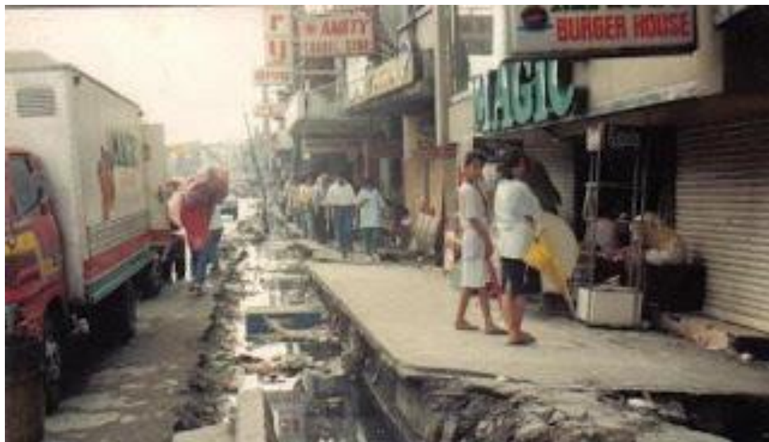
Photo No. 23.2: A photo showing roads with cracks
