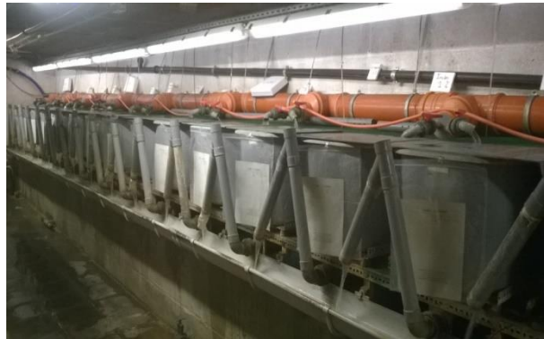
Figure 2B: Treatments tanks
