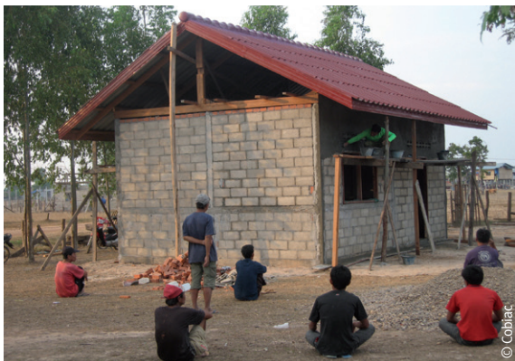
Le chantier touche à sa fin au village / The construction draws to an end at the village.
