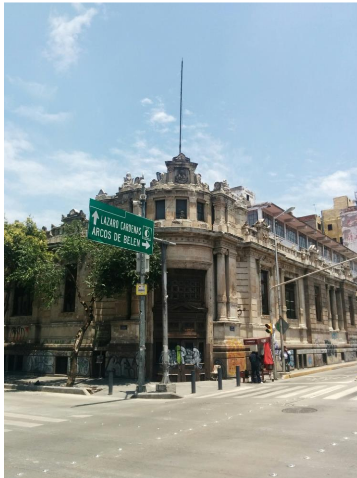
FIGURE 8. THE MAIN DOOR OF THE AHA, SUNKEN AS A RESULT OF GROUND SUBSIDENCE IN MEXICO CITY
