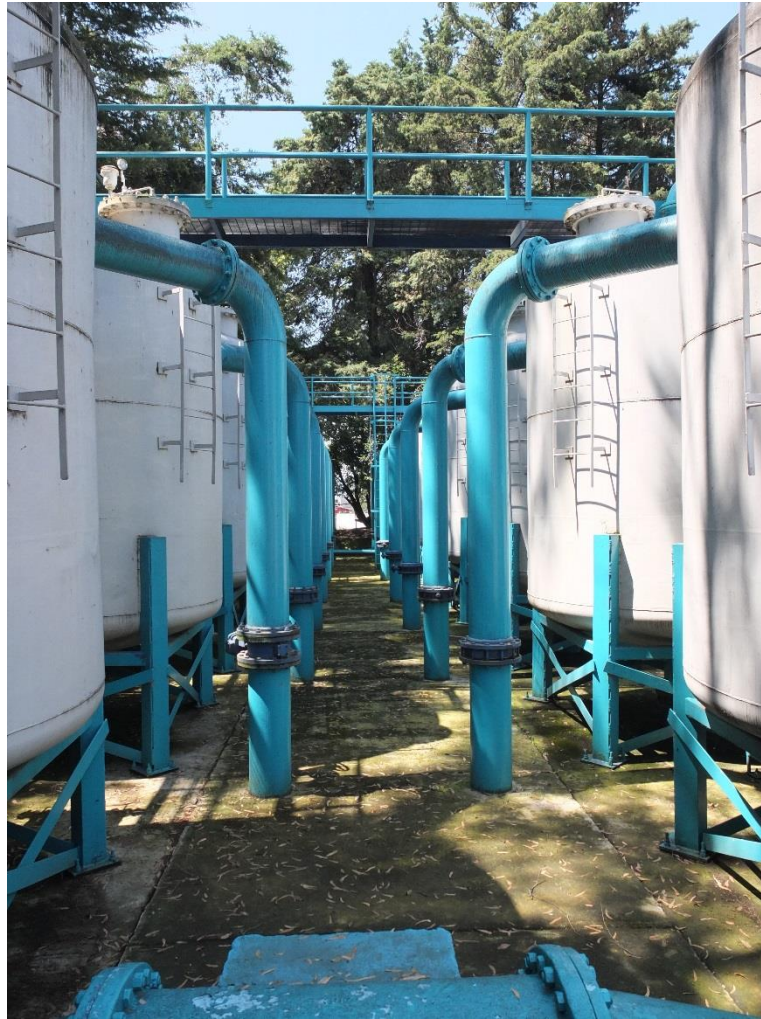
FIGURE 15. MAKING WATER PRODUCTION (IN)VISIBLE. PURIFICATION TANKS IN LERMA
