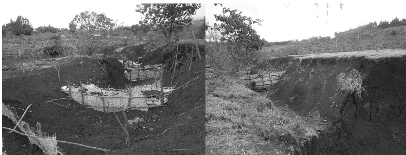
Figure 1. Check dams in the Debre-Mewi watershed, Ethiopia. Left: newly constructed check dams to stabilize a gully. Right: gully head-cut migrating towards upstream check dams.
