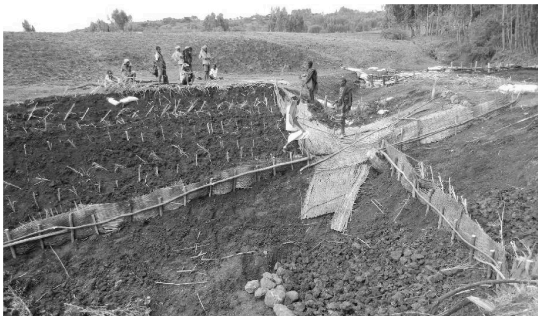
Figure 7. Construction of gully erosion control measure in the Debre-Mewi watershed, Ethiopia. Erosion control consists of regrading the gully head cut and sidewalls to approximately 40-45 degrees and protecting the soil surface with bamboo sheets and vegetation.
