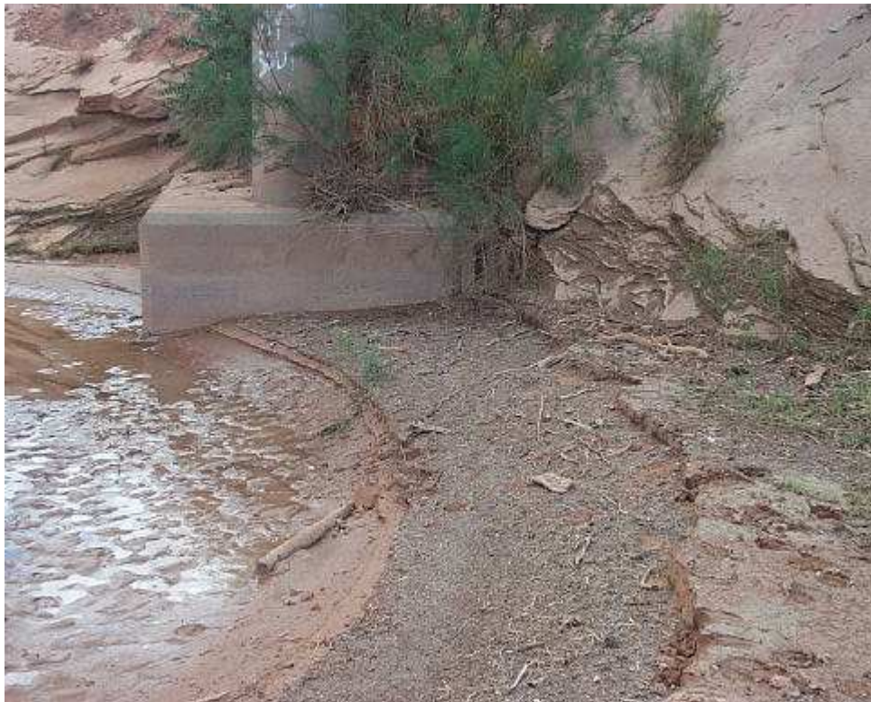
Figure 1 The scoured spread footing foundation prior to installing the countermeasure
