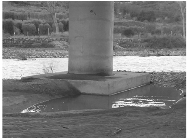
Figure 1. River Basento (Italy): Local scour around the plinth of a pier founded on piles
