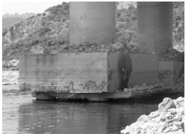
Figure 2. River Basento (Italy): General scour around a pier with consequent exposure of the piles
