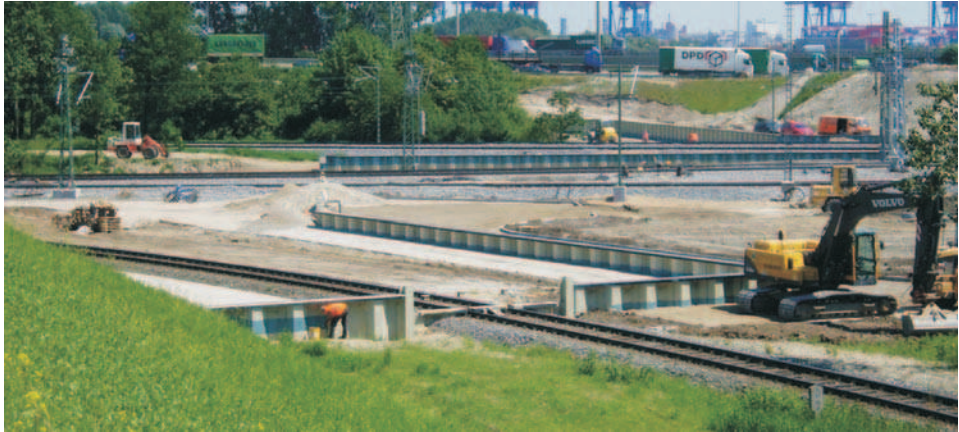
Fig. 9: Use of different protection gates (bulkhead gate in front and revolving gate, rear) at Dradenau main dike along the northern head of the port railway station “Alte Süderelbe” as part of the public storm surge protection (photo: HPA, 2006)
