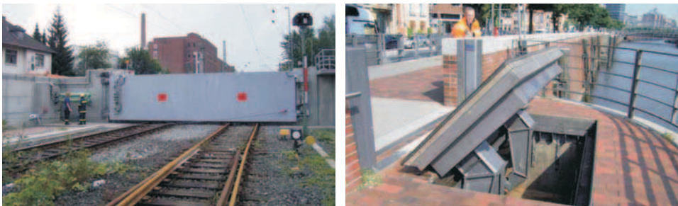
Fig. 8: Use of a flood protection lift gate (left side) and a flap gate for flood protection (right side) as part of the public storm surge protection (photos: LSBG, 2007)
