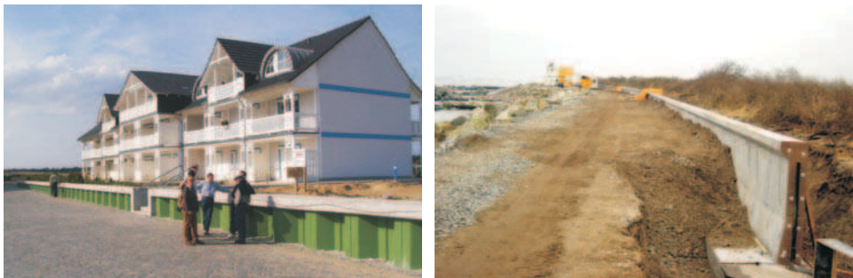
Fig. 4: Sheet pile wall with concrete cap (Karlshagen, left; length: 183 m) and cantilever retaining wall (Heiligendamm, right)
