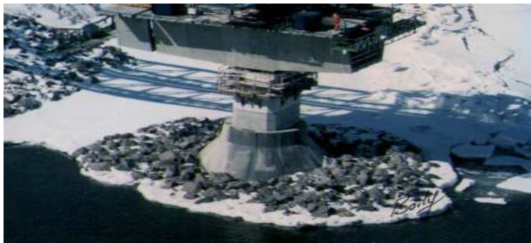
Figure 9 – Armour Stone Scour Pad at Shallow Water Approach Pier (photo by Boily)
