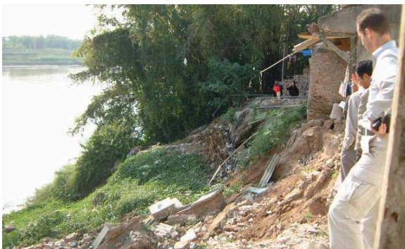
Figure 14. Damage to a house due to a sliding
