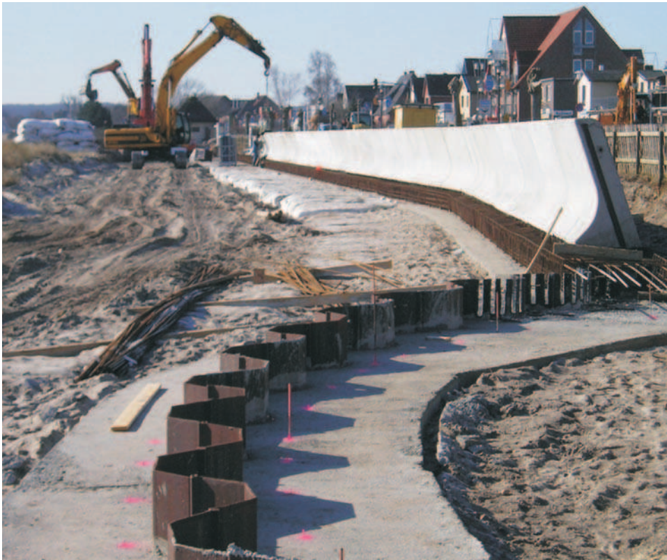
Fig. 8: Sheet pile walls mounted with concrete holms and fronted by sand containers
