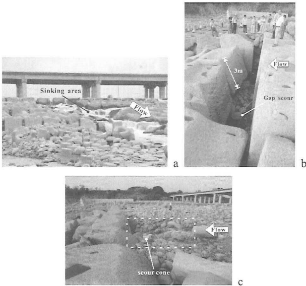
Fig 2 Failure of stepped concrete block grade control structure located downstream of Highway No.1 in Ta-Chia River in central Taiwan (November 2009): (a) blocks tilting and sinking; (b) deeper scour depth than block height; and (c) a scour hole upstream of the sinking area
