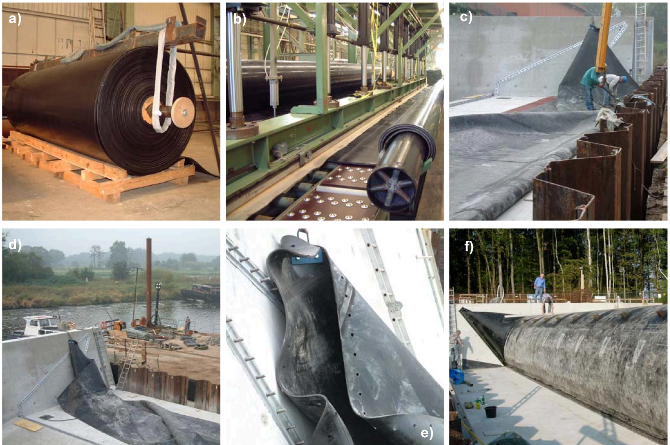
Figure 1: Weir Marklendorf on the River Aller: a) Membrane after calendaring b) Joining the sheets c) to e) Installing the rubber membrane in October 2005 e) Pressure test
