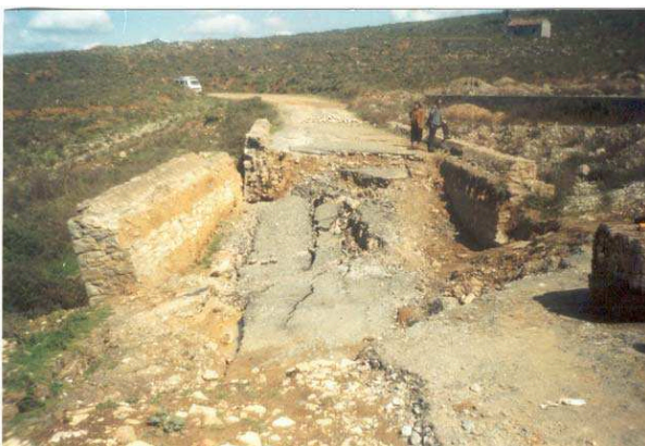
Photo nr. 5. Kallmeti bridge. It's looking to north, and shows, the sinking of its pillars and pavement
