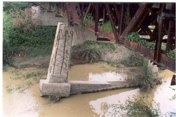
Photo nr. 4. Mifoli bridge. It's looking to north, and shows, the sinking of its pier
