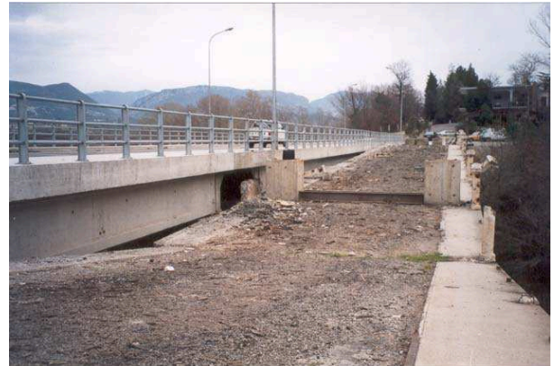
Photo nr. 2. Peshkatari bridge. It's looking to south, and shows, the new bridge and the destroyed bridge (right side) which is sunken 1.98 m compared with the new bridge.
