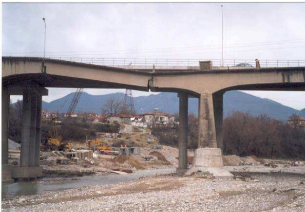
Photo nr. 1. Peshkatari bridge. It's looking to east, and shows, cracks, destroyed beam and a sinking of pier.
