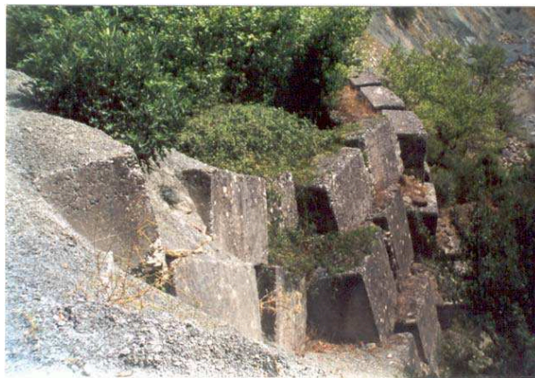
Photo nr. 7. Bogova landslide. It's looking to east, and shows, a destroyed retaining wall (deformed) by mass movement
