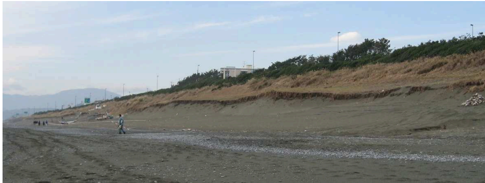
Fig.3 Vegetation area eroded by storm waves (at Fig.2 , #2)
