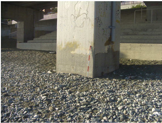
Fig.7 Eroded beach around Kozu (Fig. 2, #4).
