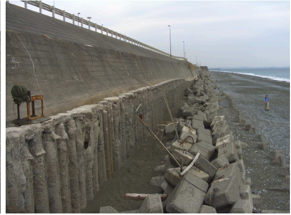
Fig.6 Damaged sea wall at Oiso (Fig.2, #3)
