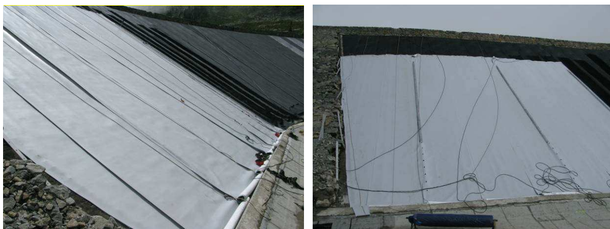
Figure 7 and Figure 8 Left: Geomembrane sheets are being unrolled from crown to articulation joint. Right: The upper \Omega -shaped profile is installed over two overlapping adjacent sheets.
