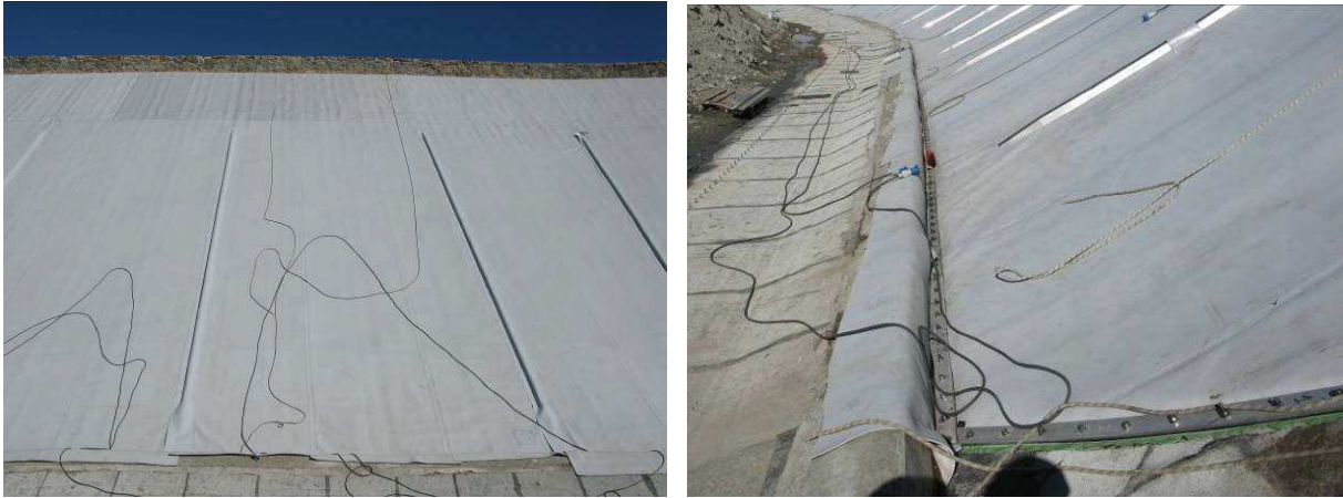
Figure 9 and Figure 10 Left: geocomposite strips welded over the upper \Omega -shaped tensioning profile. Right: view on the perimeter watertight seal at the articulation joint.
