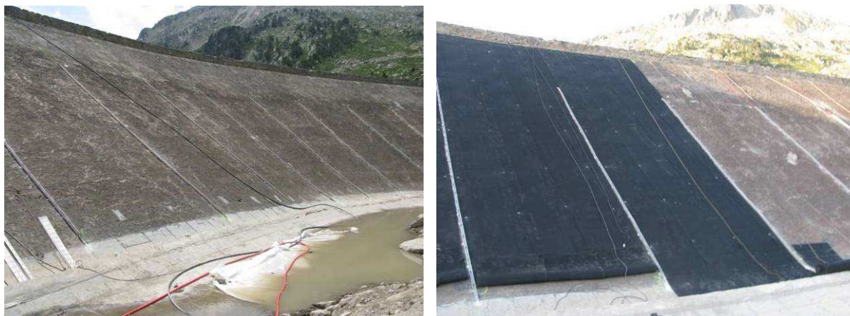
Figure 5 and Figure 6 Left: view on the U-shaped tensioning profiles mechanical fixed via chemical anchors to the concrete facing. Right: view on the geonet sheets being laid down between lower tensioning profiles and mechanical fixed via impact anchors to the concrete subgrade.
