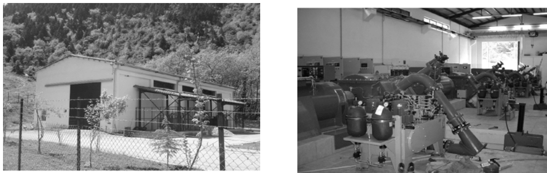
Figure 6 The common powerhouse of the Small Hydropower Plants of Krya Vrissi and Triantafyllia with 4 in total turbines
