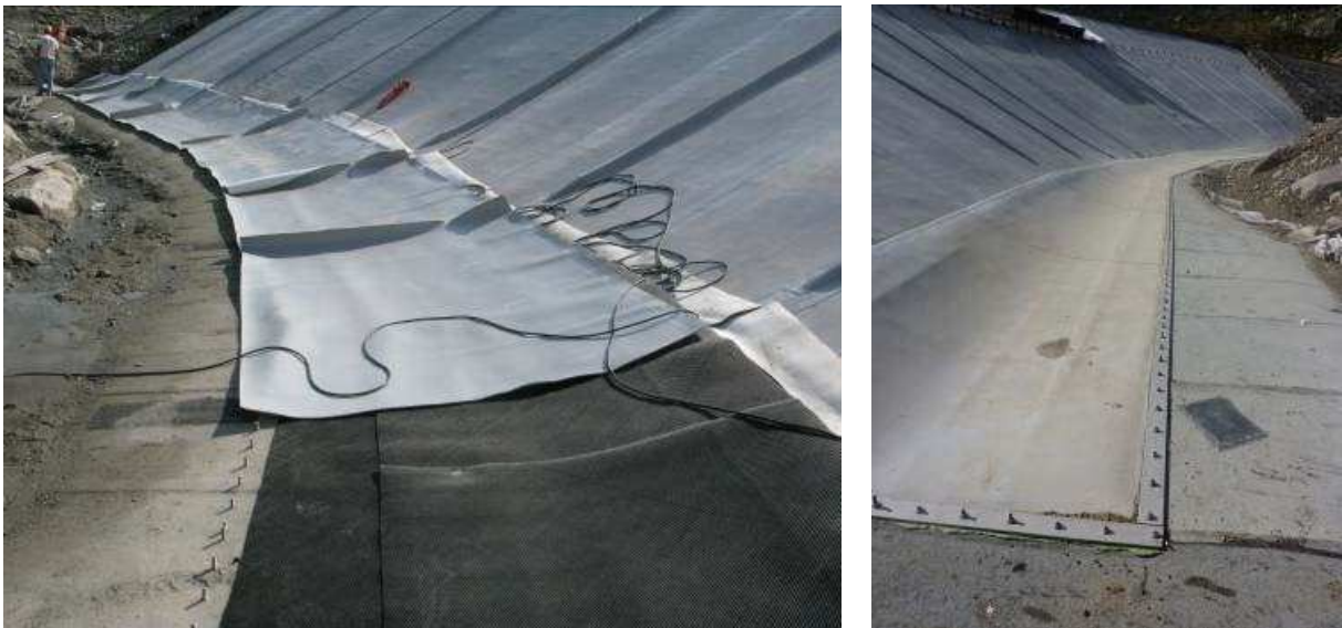
Figure 11 and Figure 12 Lower section from articulation joint down to toe. Placement of the geocomposite sheets over the drainage geonet, and the secondary perimeter seal completed.
