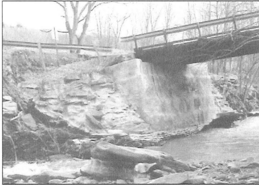
Figure 4. This photo illustrates the importance of embankment strength with respect to the development of abutment scour: the slope failure of the embankment immediately behind a wing-wall abutment founded on a spread footing.
