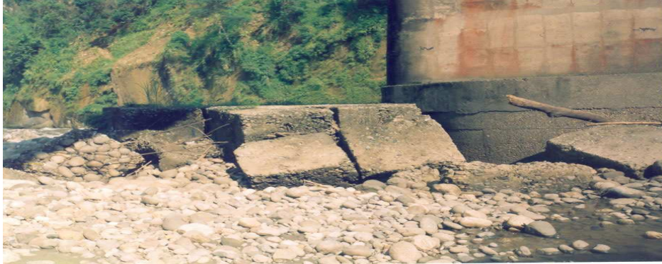
Fig 4 Scour around pier
