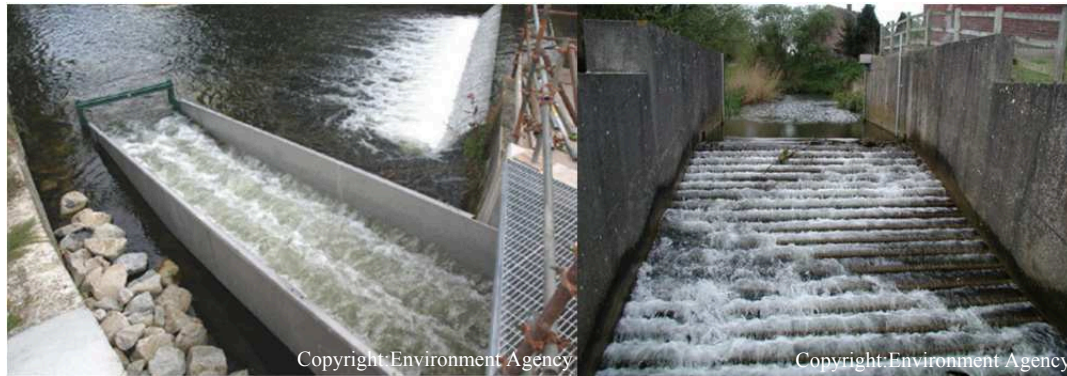
Figure 2: A Larinier fish pass on a flow gauging weir (left) built to ISO 26906:2009 and Low Cost Baffles (right) designed to ISO/AWI TR 19234
