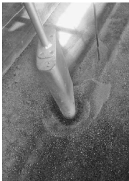
Figure 10. Photograph showing scour around round nosed pier
