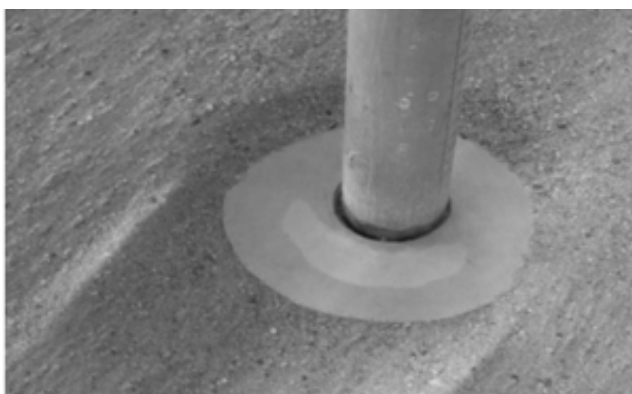
Figure 2. Photograph showing scour around the pier fitted with collar
