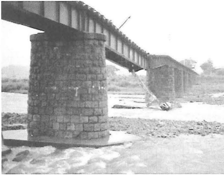
Figure 1 Destructive effect of scouring under a railway bridge (Japan).
