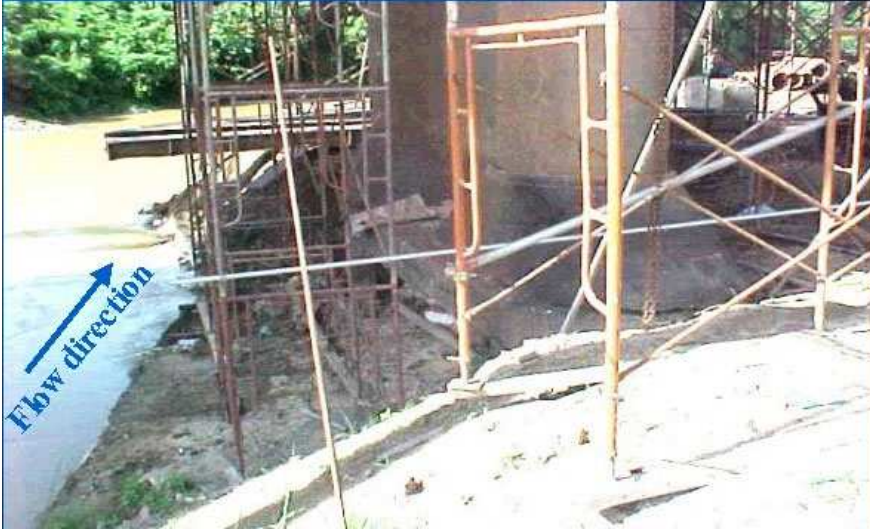
Fig. 1. Abutment scour at Muda River in Jediang, Malaysia (Photo courtesy of Shanker Kumar Sinnakaundan, River Engineering and Urban Drainage Research Center, Malaysia)
