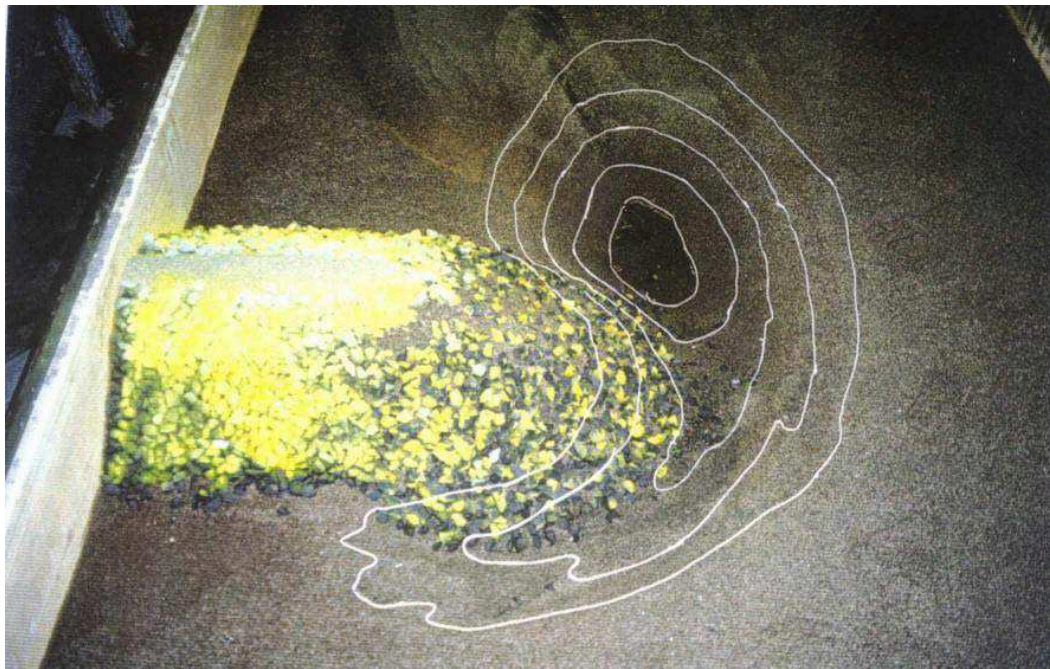
Figure 5 – Typical scour hole developed at an abutment (of no failure) with riprap protection, viewed from downstream
