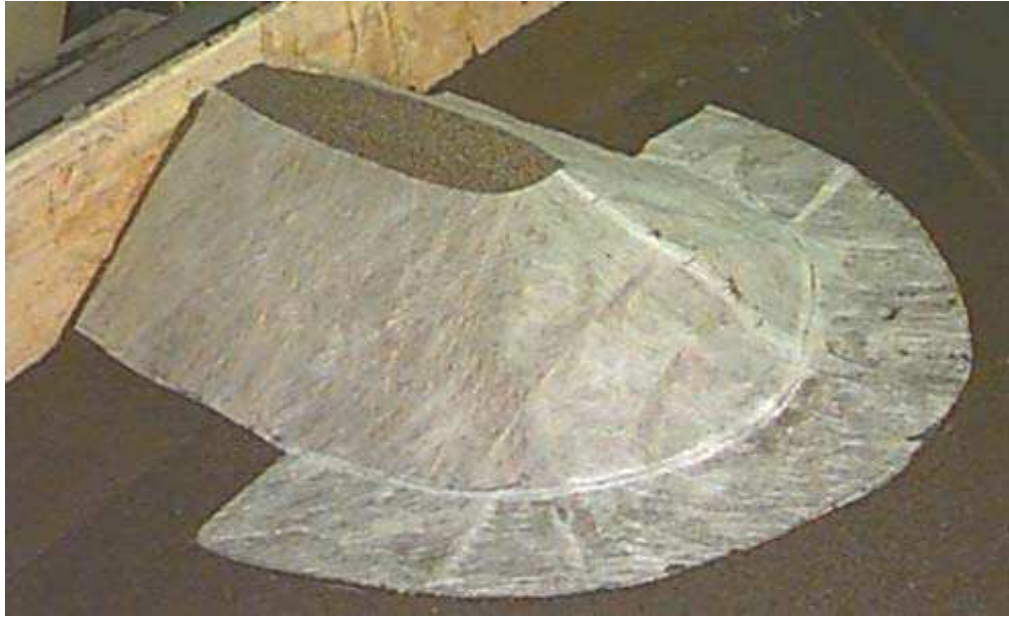
Figure 4 – The filter fabric placed over the sand embankment ready for placement of cable-tied blocks
