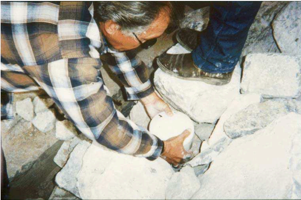
Figure 5. Installation of a float-out device to monitor riprap stability. (Lagasse et al, 2001)
