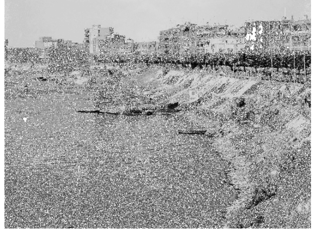
Figure 13 Protected bank in river bend at Kafr-el-Zayat (Rosetta branch) just downstream of the railway bridge (right bank)
