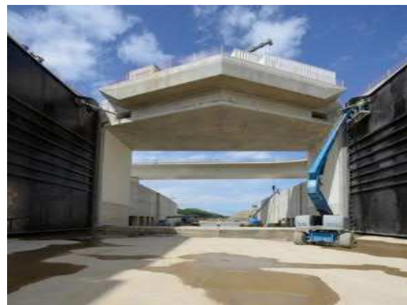
Fig.6: Downstream mitre gate – © JL DERU/photo-daylight
