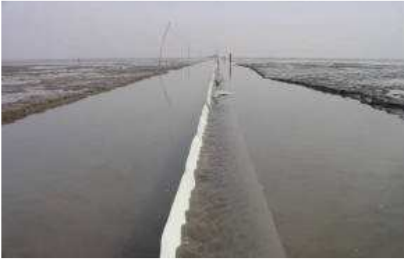
View of pipeline at shore approach during low tide. Note that minor rotation had occurred during pulling operation, partially due to flooding and receding tides. Note scour on both sides of pipeline due to spoiler effects.
