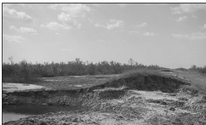
Figure 8. Overtopped levee in New Orleans (source: ILIT, 2006)
