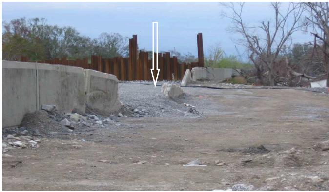
Figure 10. Piping failure in New Orleans
