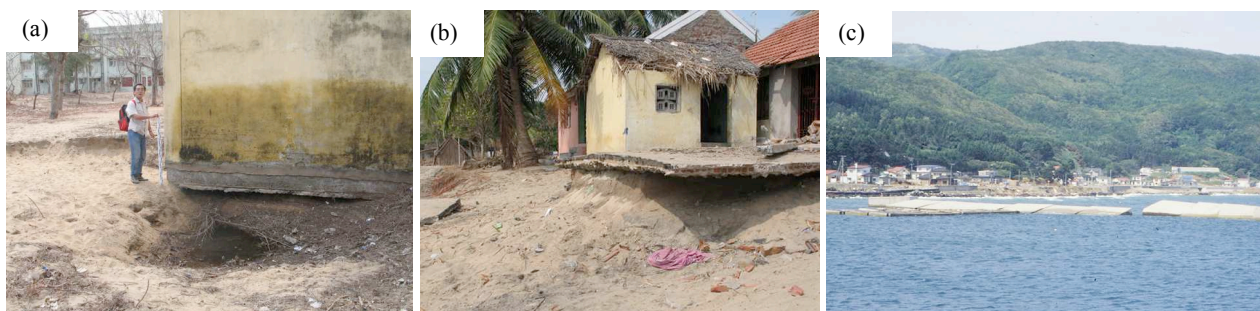
Figure 1. Typical scour holes at building foundation: a) approximately 1.5 m deep in India, 2004 tsunami (photo by Yeh); b) 1.4 m deep in India (photo by Yeh, PI); c) foundation failure of the breakwater by the tsunami (Okushiri, Japan, 1993; photos by Yeh).
