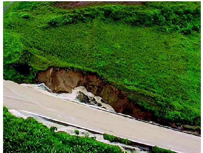
Figure 3: Close up view of principal failure area (Source: Hidroven)
