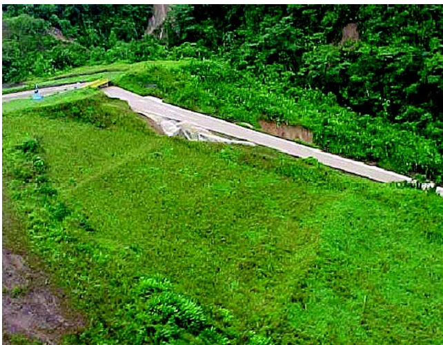
Figure 2: Lined spillway channel failure commences (Source: Hidroven)
