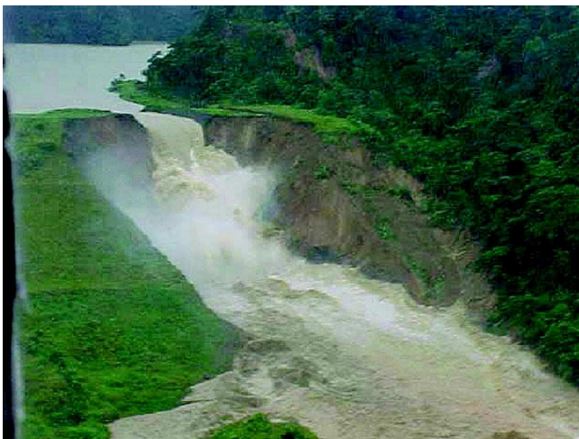
Figure 4: Advanced level of failure, showing headcutting mechanism (Source: Hidroven)
