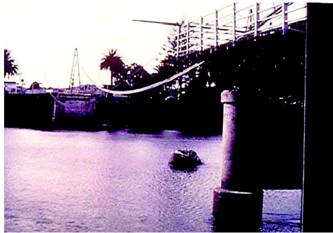
Figure 6: The damaged Wairoa River Road Bridge, flow from left to right, after Melville and Coleman (2000)
