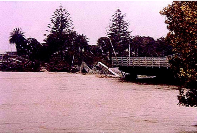
Figure 7: The bridge failure, flow from left to right, after Melville and Coleman (2000)
