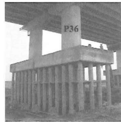
July 2009 (piles exposed around 7.5m)
