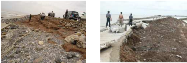
a. damage of armour layer and erosion upper part of outer slope b. Damages of crest-wall and erosion of inner slopes
