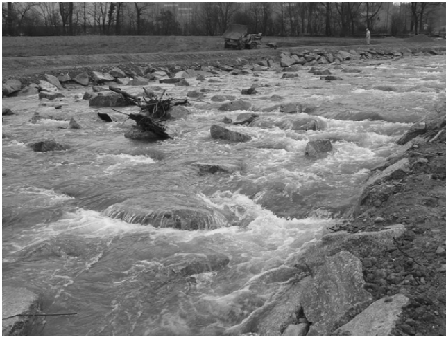
Figure 5. Ramp type B with unstructured blocks at the Wyna River (Canton Aargau, Switzerland) with a specific discharge q of about 0.16 \text{ m}^2/\text{s} (view against flow direction). Source: Hunziker Zarn & Partner.
