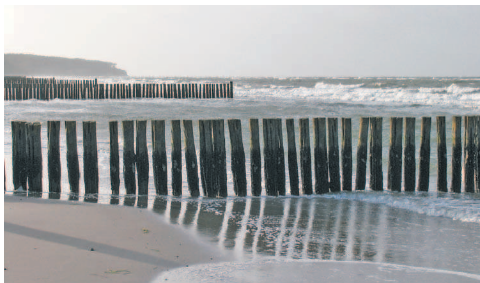
Fig. 1: Wooden single-row pile groynes at low water at the Baltic coast near Warnemünde (photo: WEICHBRODT, 2006)
