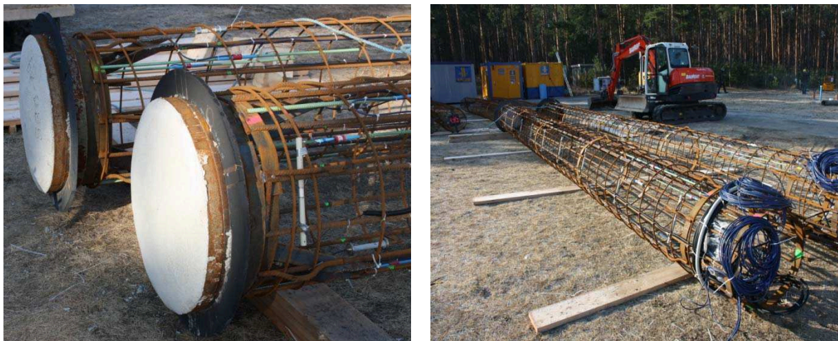
Figure 5: Reinforcement cages of piles P1 and P2 with instrumentation. Toe load cells and various strain gage, fiber-optic and ultrasonic sensors can be seen on the left.
