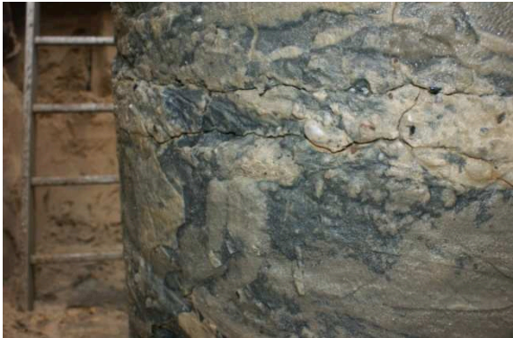
Figure 11: Pile P7: Left: excavated pile. Top. Cracks at 3.75 m depth below top of pile.
