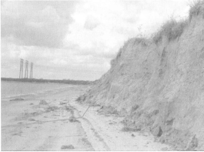
Figure 4. Picture of Phase One embankment after Hurricane Jeanne.
