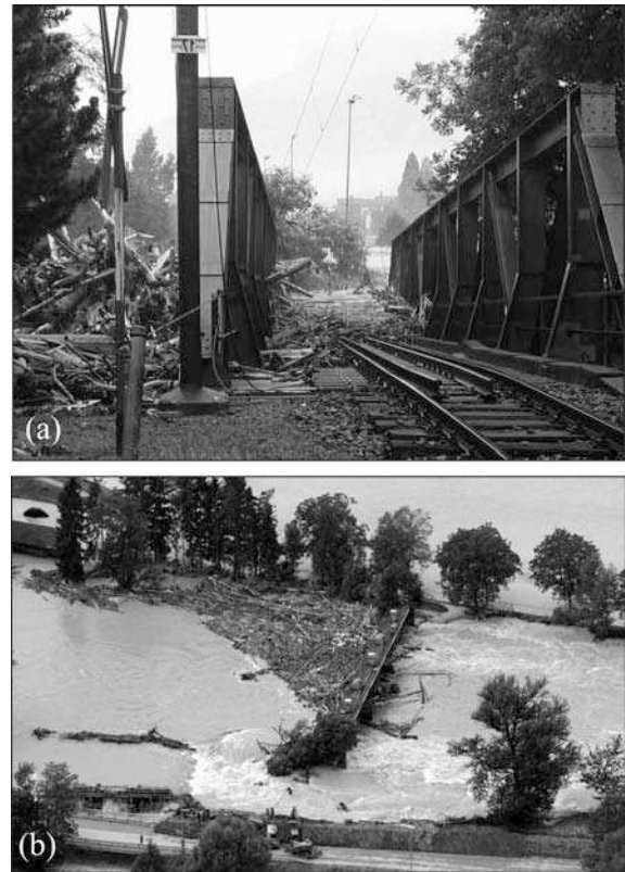
Figure 1. Drift accumulation at (a) railway bridge in Sarnen and (b) weir Perlen in Lucerne, during 2005 flood event in Switzerland, flow direction from left to right
