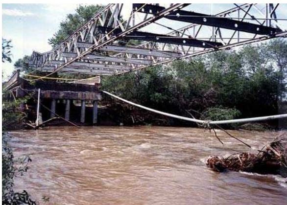
Figure 7: Looking downstream at Bailey Bridge Launching in March, 1995 (photo by Steve Ng, Caltrans)
